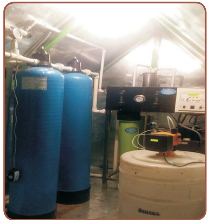
Reverse Osmosis Plant
