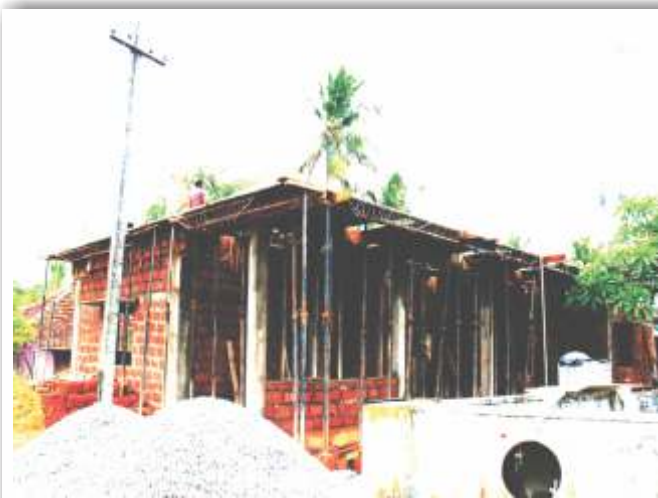
Construction work in progress for new school building at DKZP Higher Primary School, Tannerbaavi, Panambur, Mangalore.
