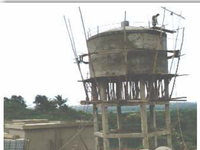
50000 Ltrs capacity water tank under construction by KIOCL for the resettlement Colony at Porkodi
