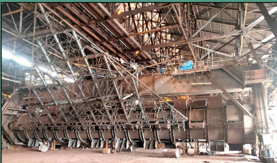
[View of Blender Reclaimer]
