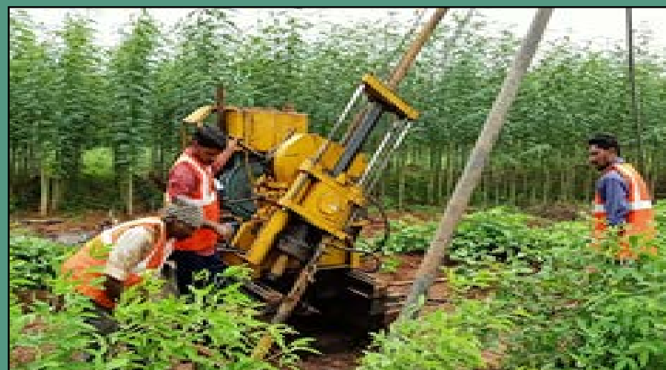
[Drilling works carried out at UDBUR BLOCK, MYSORE (Dist), KARNATAKA allotted by Ministry of Mines, Govt for establishing Nickel and Chrome zones.]
