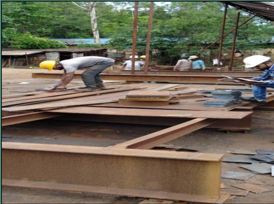
[A view of the fabrication and installation work at M/s OMC at South Kaliapani]
